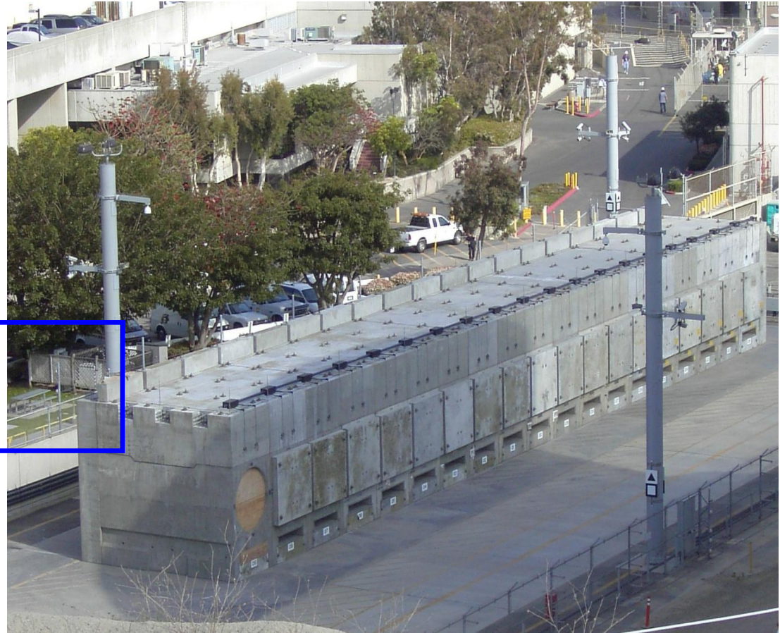
Southern California Edison – SONGS Units 1, 2, and 3
