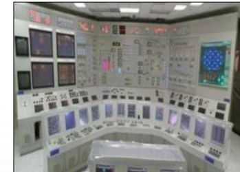
Instrumentation and Control
