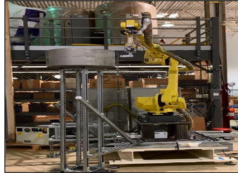
Canister decontamination robot arm
