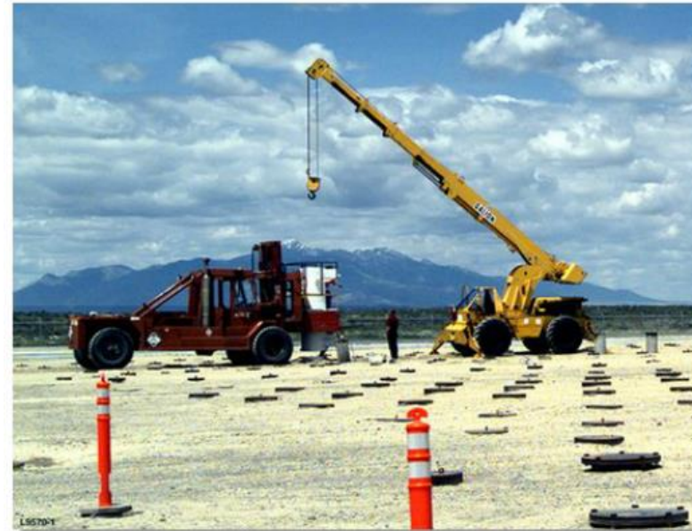
Waste package loading at RSWF, MFC-771
