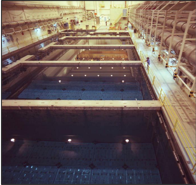
CPP-666 fuel basin
