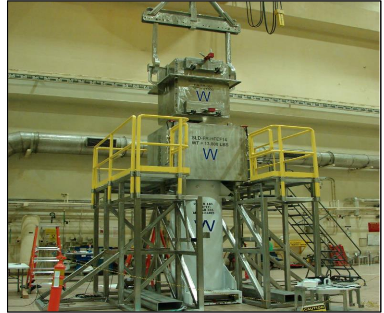
HFEF-14 Fuel Transfer Cask
