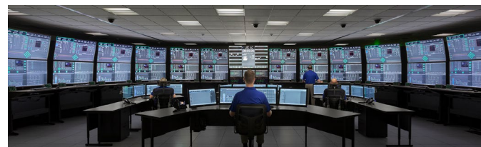
NuScale Control Room Simulator
