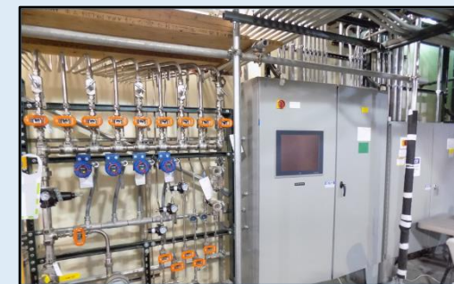
Wet decon system control station
