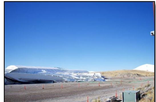
ARP IV structure collapsed
