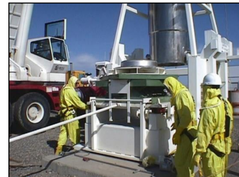
Spent fuel storage facility
