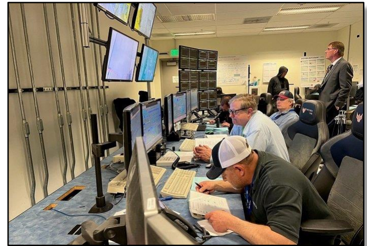
IWTU control room – startup of sodium bearing waste operations on April 11, 2023
