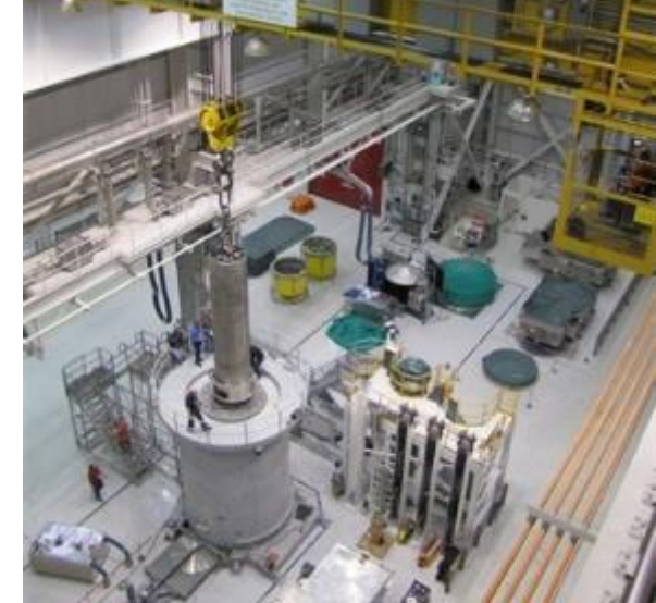
Spent Fuel Packaging Facility
