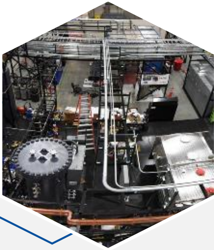
25 kW High Temp Electrolysis Stacks V&V
